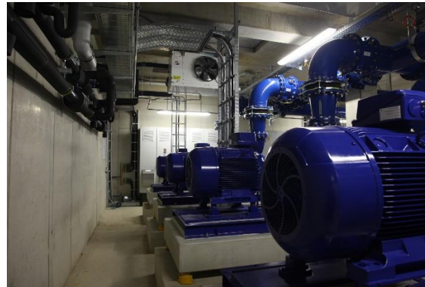
4 x 250 l/s (80 kW KSB-Pumpen)
